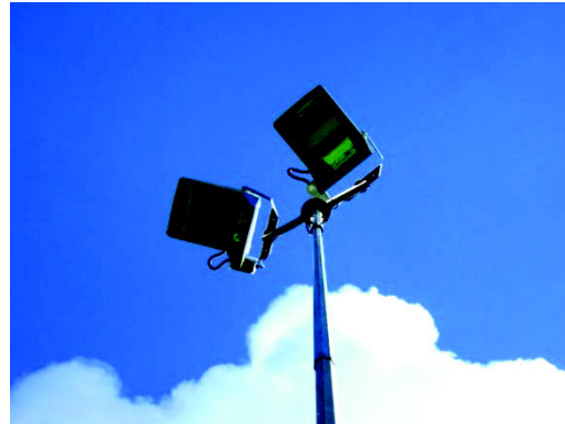
Example of floodlight mast mounted with two luminaires c/w 2kW lamps / fitting
