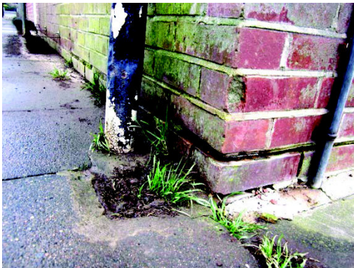
Damaged pointing requires rectification
