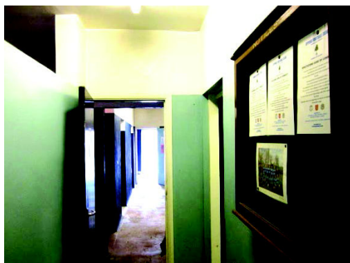
Inadequate emergency provision
