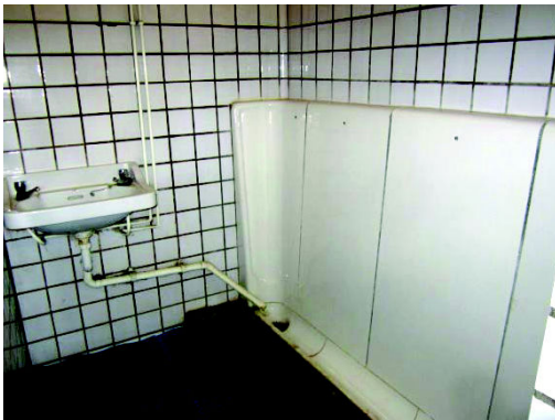
No water supply to urinals
