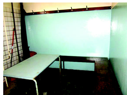
No WC in referee changing accommodation
