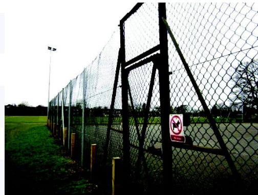
Perimeter ball-stop fencing
