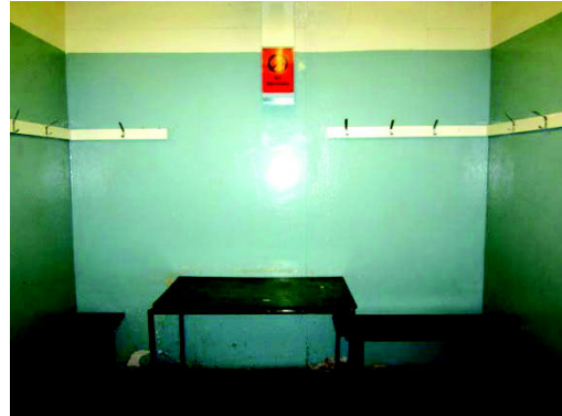
Undersized changing rooms
