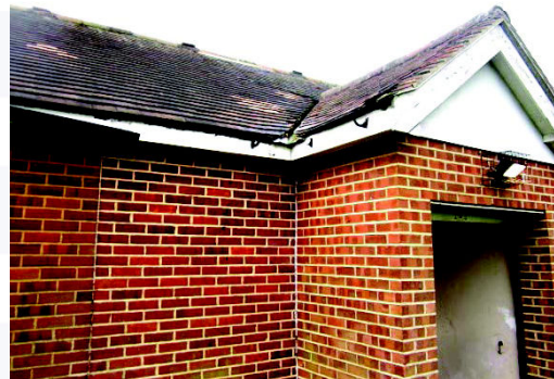
Damaged guttering requires rectification
